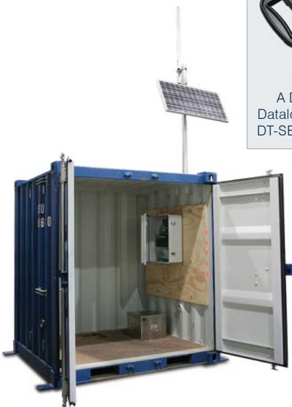
6 ft. Instrumentation House with solar panel and antenna.
