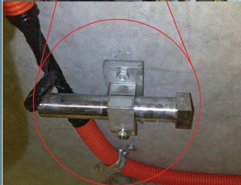
Typical installation of the RST Profile Monitoring System for Tunnel Concrete Segments with an RST flexDAQ Datalogger System. Inset photo shows close-up.
