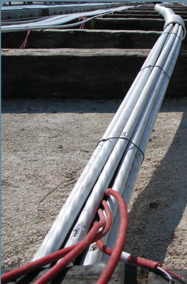
Finished multi-strand anchor with DCP (double corrosion protection) instrumented with 4 TENSMEG gauges.
