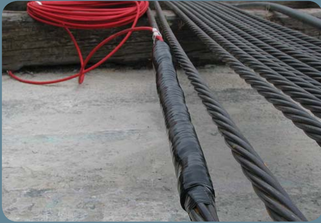
TENSMEG gauge with water proofing installed on one 7-wire strand of a multi-strand anchor.
